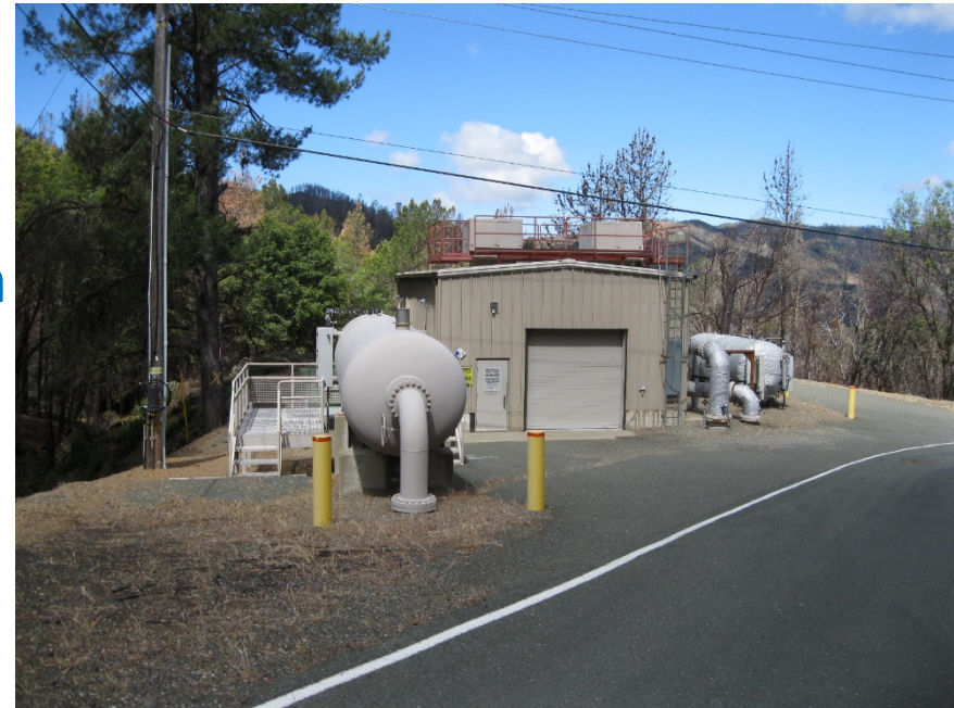
Bear Canyon Pump Station #3
