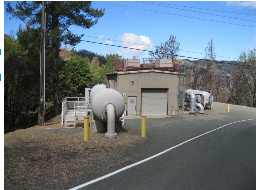
Bear Canyon Pump Station #3
